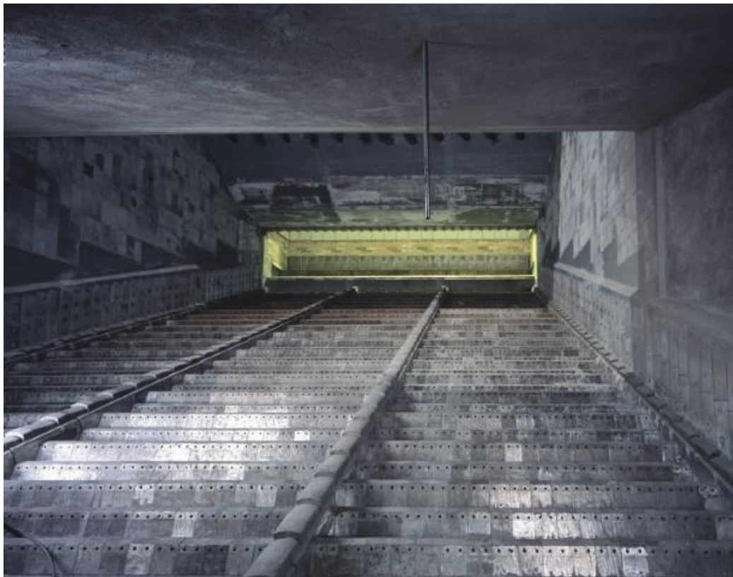
Plate 3.6: Typical Combustion Chamber and Grate
