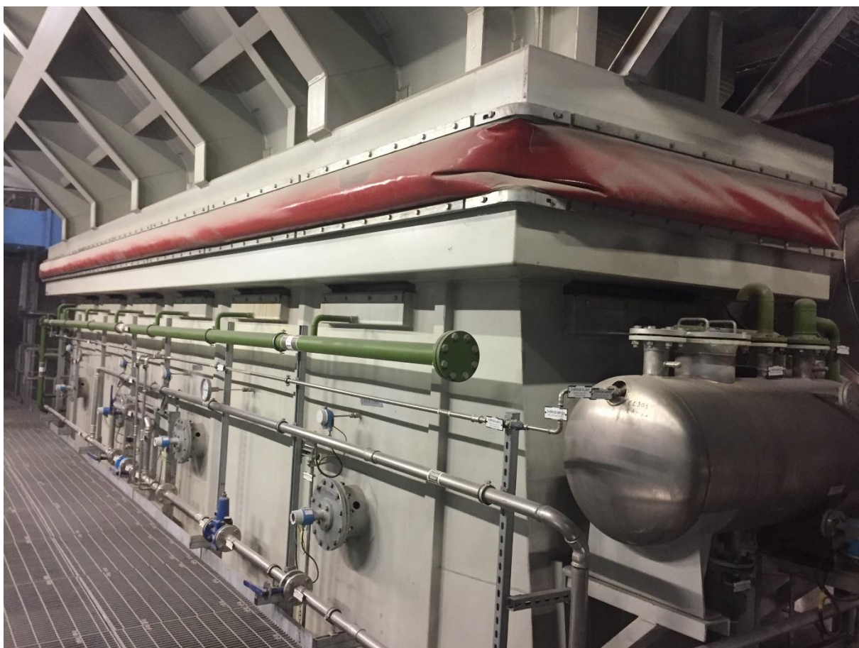
Plate 3.5: RRRF Waste Feeding Hopper
