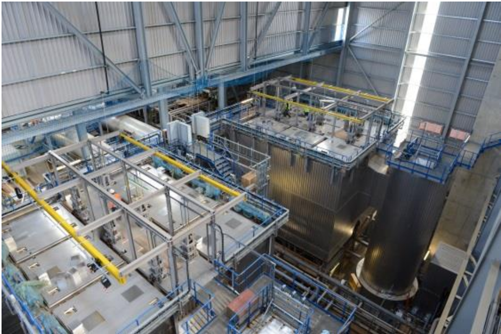
Plate 3.7: Typical Bag Filter House
